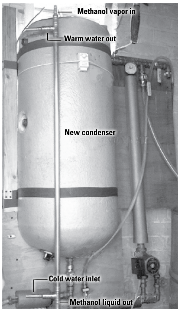
FIGURE 10. CONDENSOR ON BIODIESEL REACTOR.
